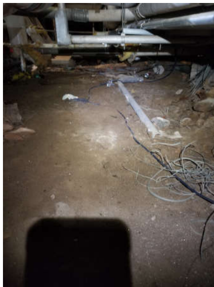
crawl space 3 debris 3
