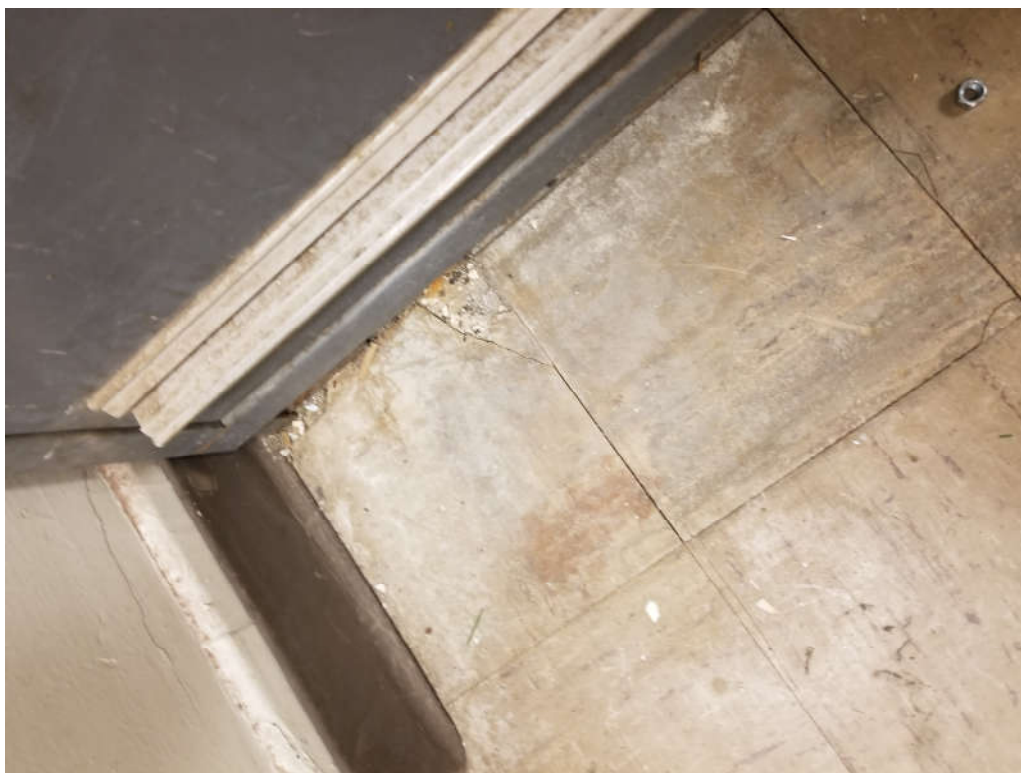
room b28 9x9 floor tile cracked tile
