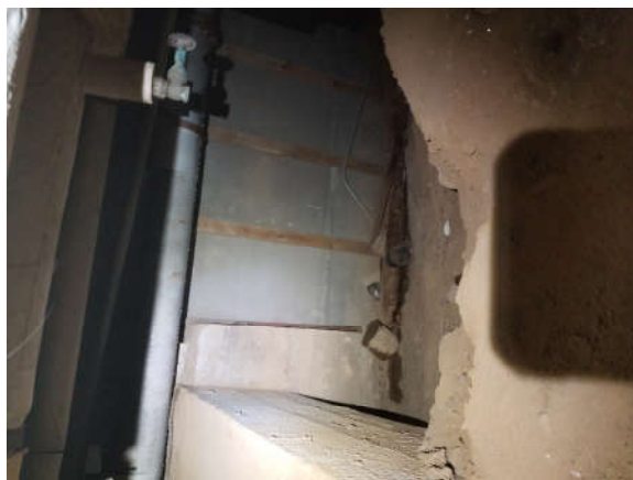
crawl space 3 transite 2
