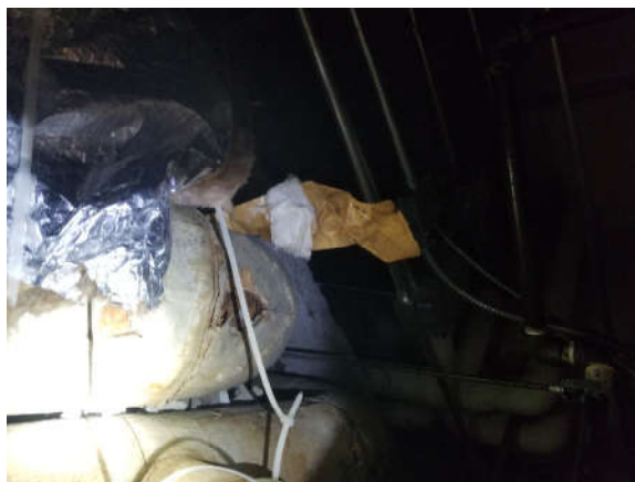
room b430 damaged fitting
