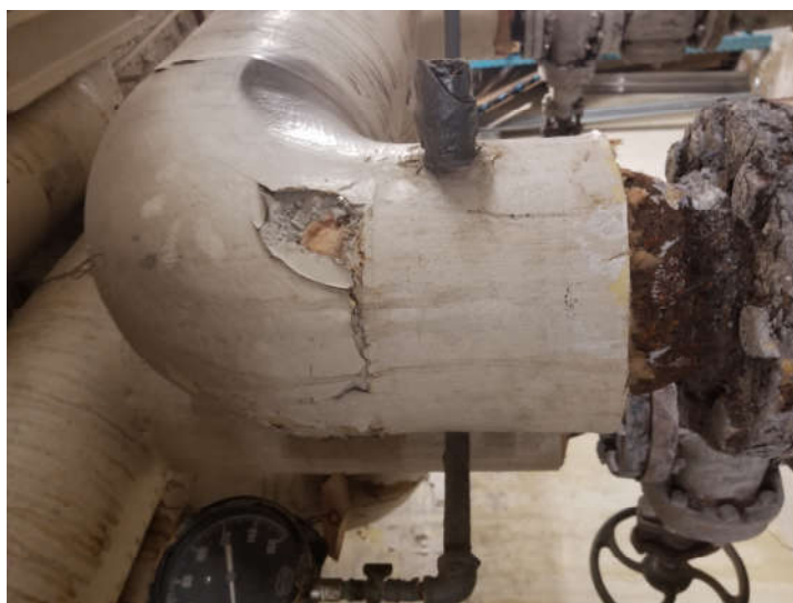
b-2 storage area damaged fittings
