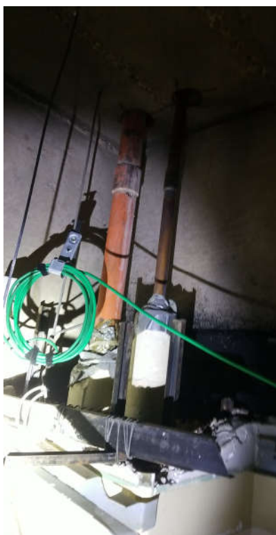
a160 pipe in wall
