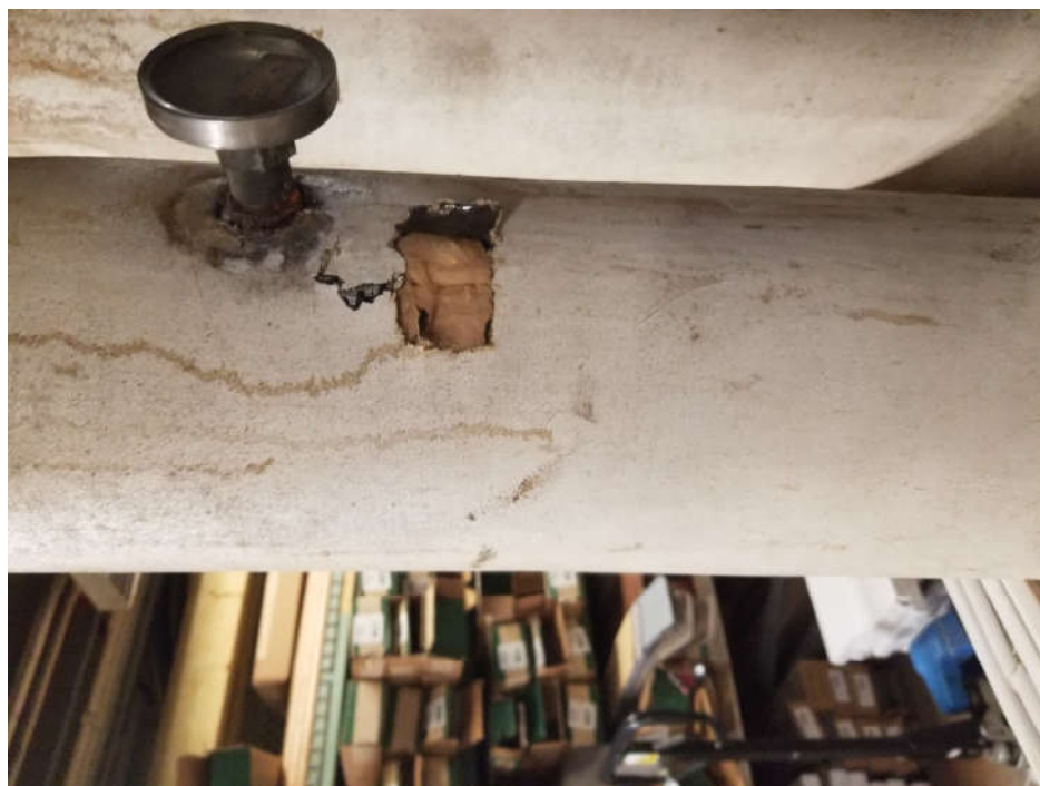
b-2 storage area damaged fittings 2
