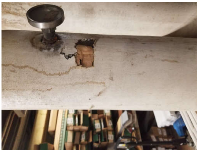
b-2 storage area damaged fittings
