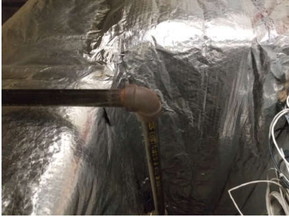
basement sprinkler thread sealant
