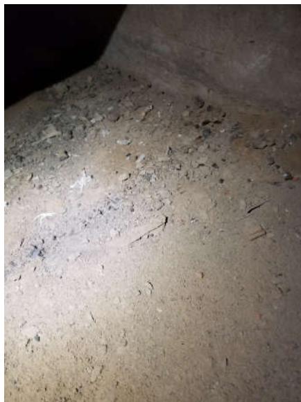
crawl space 3 debris 4
