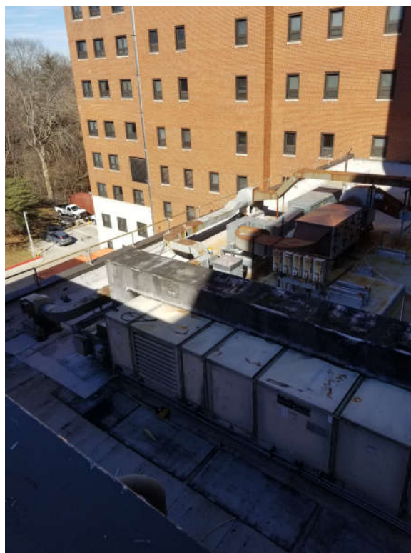
4th floor roof duct mastic 2
