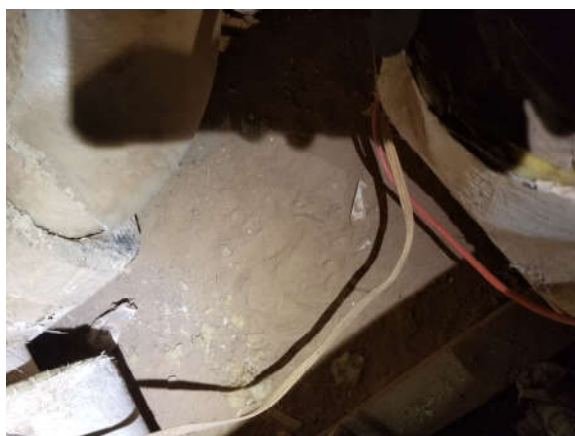
crawl space 3 debris 1
