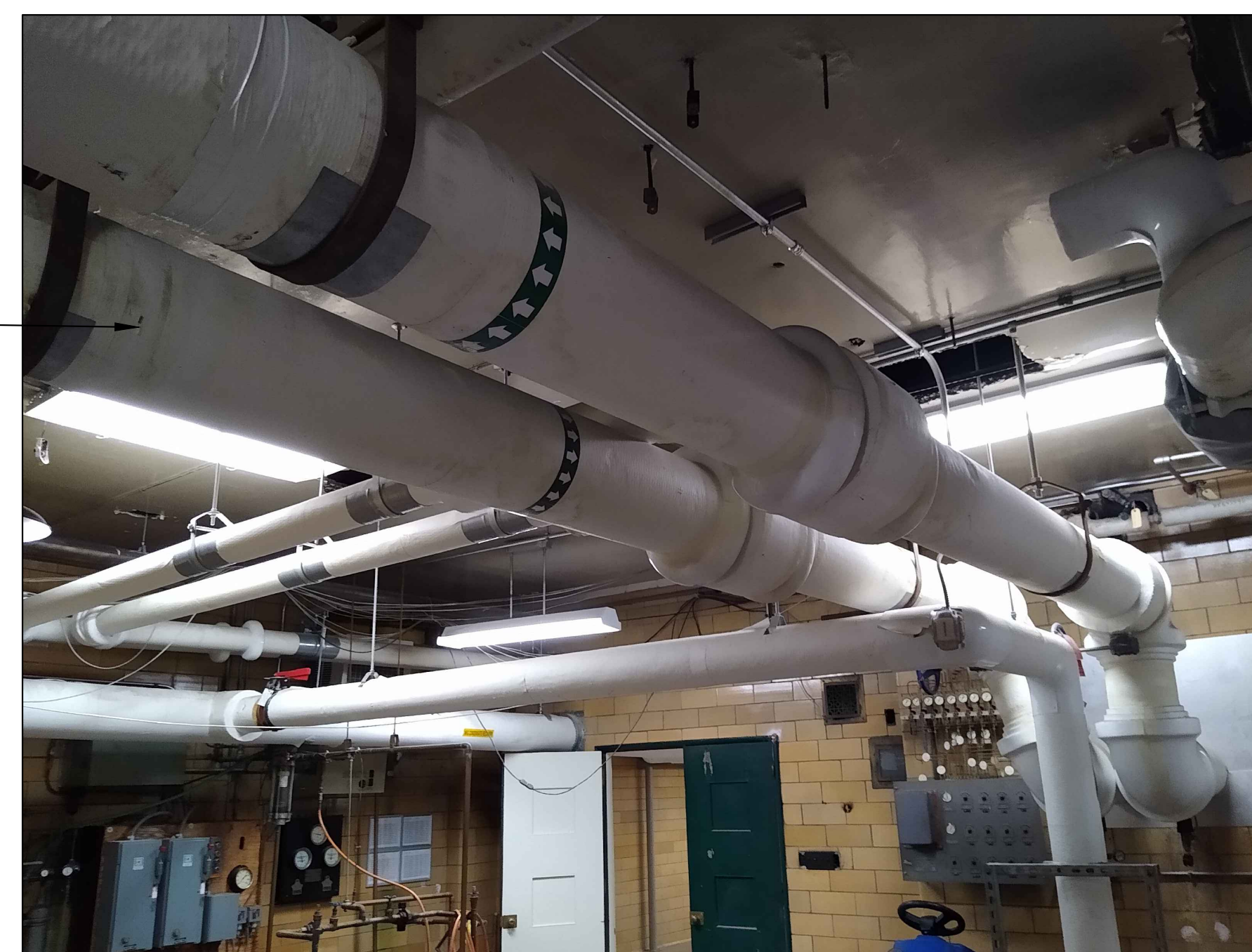
9 PHOTO: CHWS (REPLACE AS INDICATED), CHWR (REPLACE TEMP SENSOR) M-5 Scale: NONE
