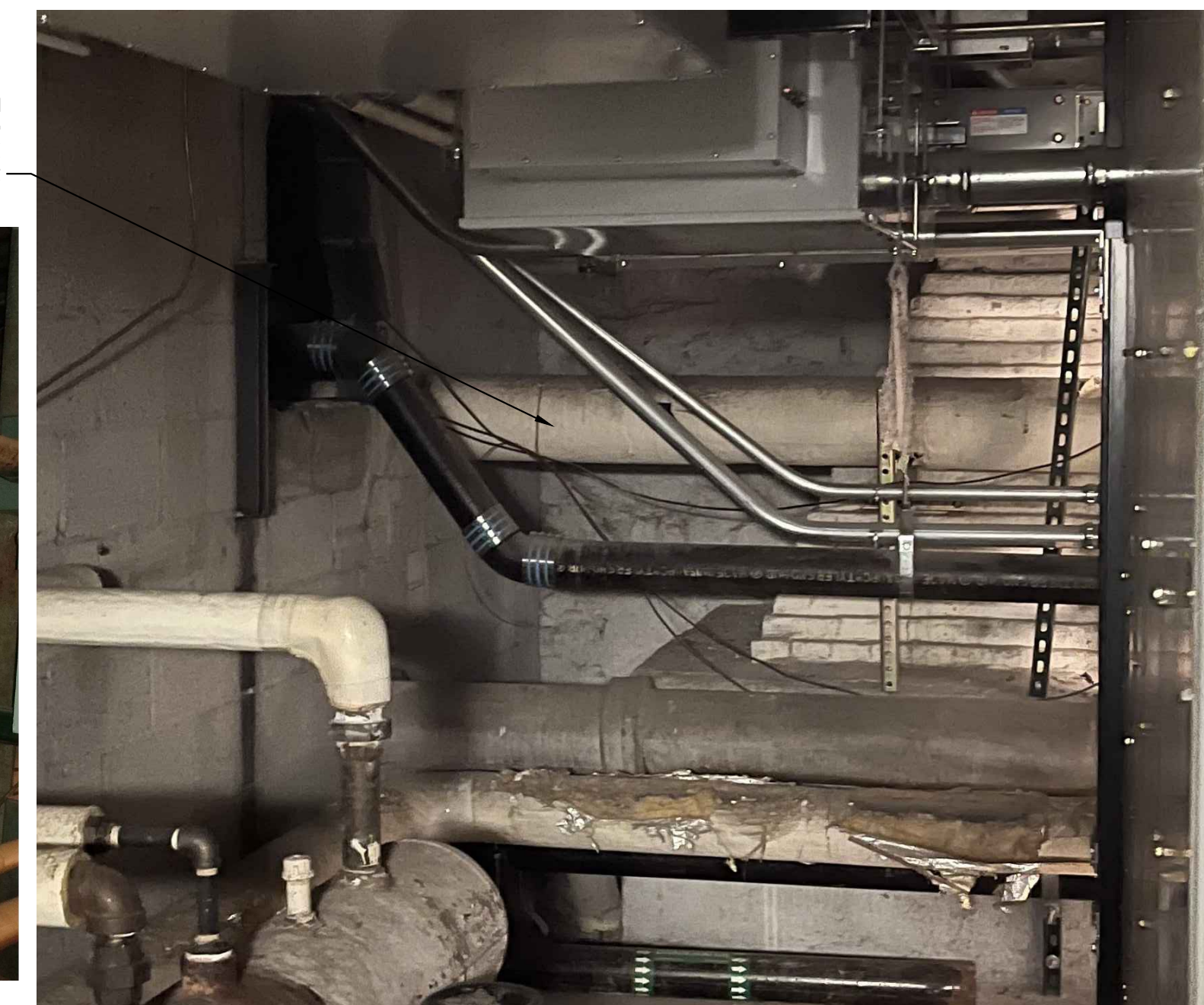
6 PHOTO: STEAM METER LOCATION M-10 Scale: NONE ALT VIEW
