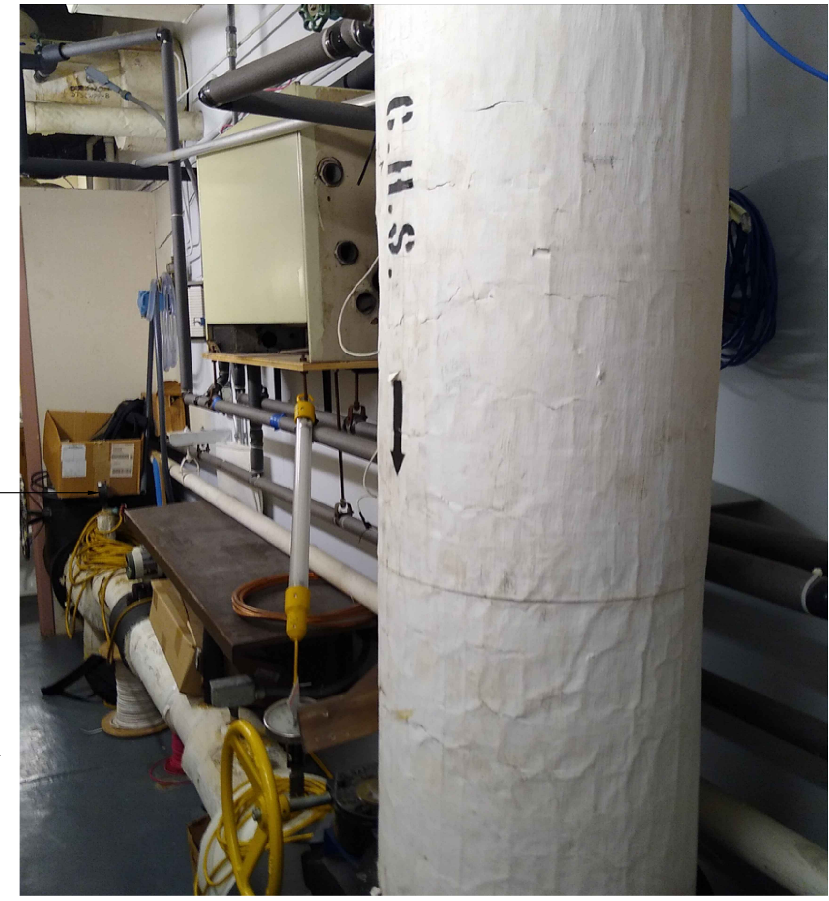
8 PHOTO: CHILLED WATER METER LOCATION GENERAL BLDG M-8 NOB-CHWS-M1
