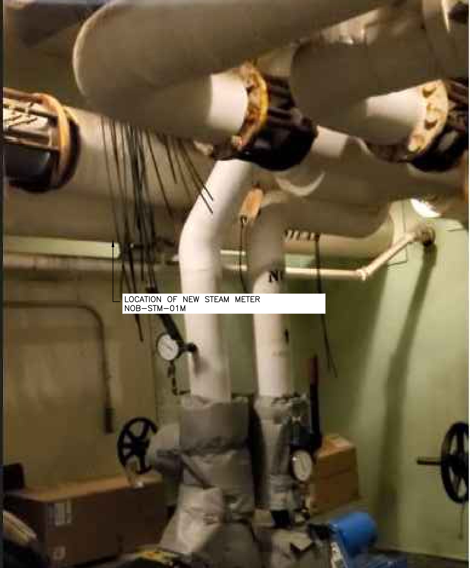
5 PHOTO: LOCATION NEW STEAM METER M-8 NOT TO SCALE NOB-STM-01M
