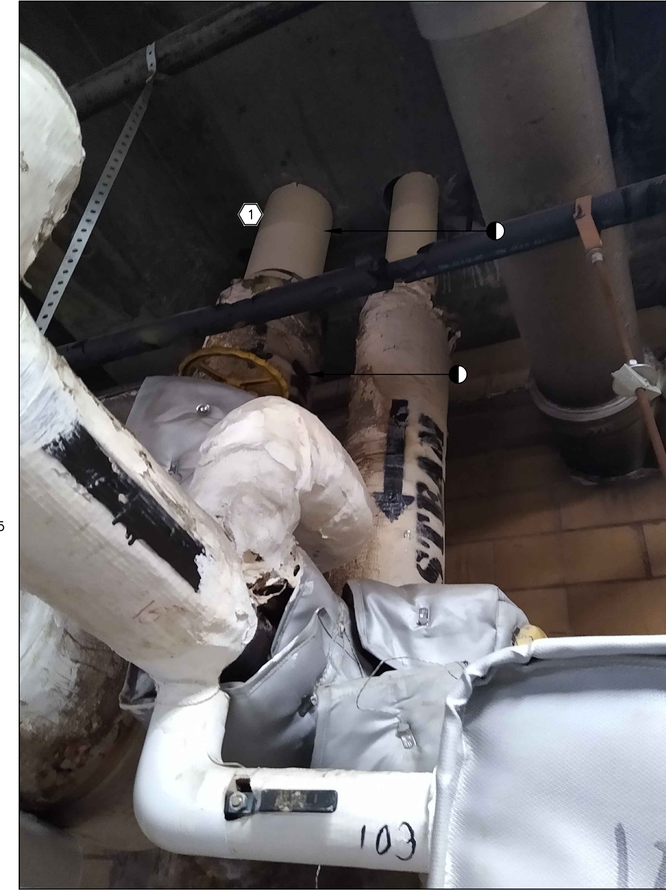
3 PHOTO: STEAM SERVICE ENTRANCE M-5 Scale: NONE LOCATION OF NEW METER
