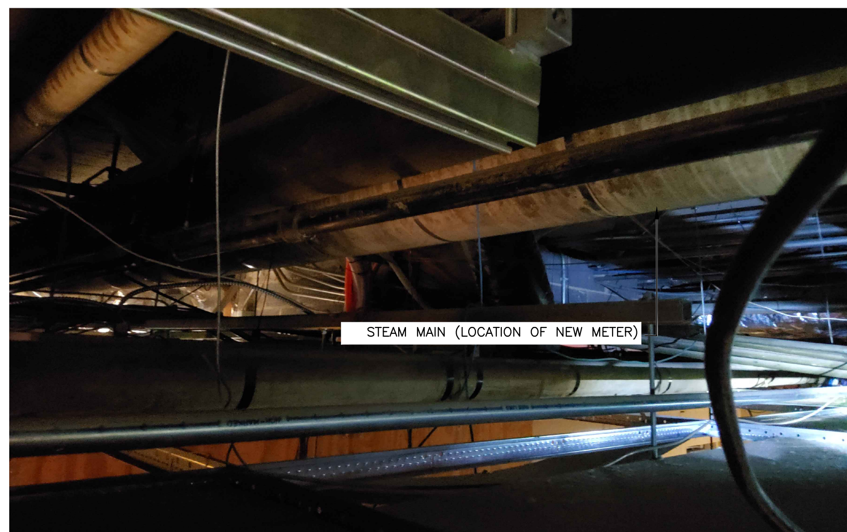
3 PHOTO: STEAM METER LOCATION Scale: NONE ABOVE CORRIDOR CEILING
