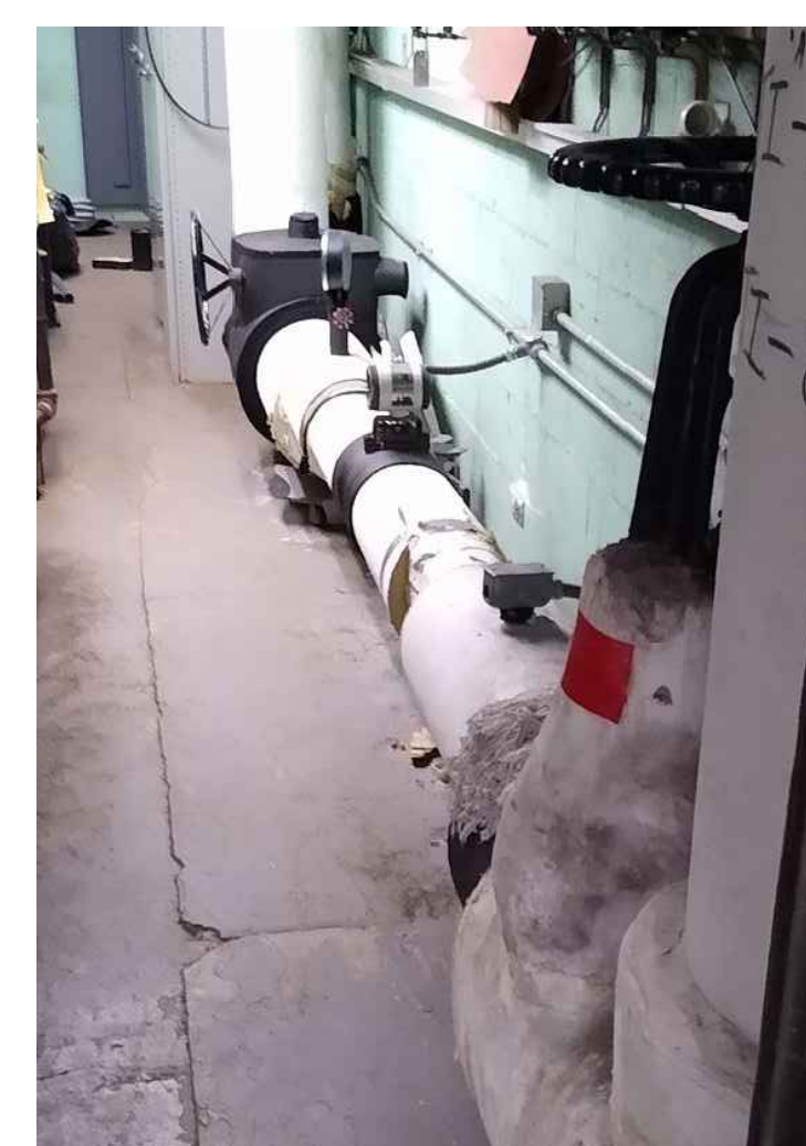
4 M-11 EXISTING CONDITIONS CHILLED WATER METER LOCATION No Scale
