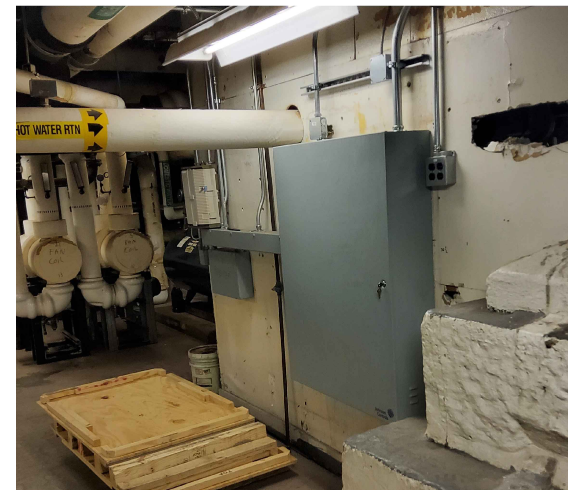
4 PHOTO: EXISTING CONTROL PANEL M-10 Scale: NONE
