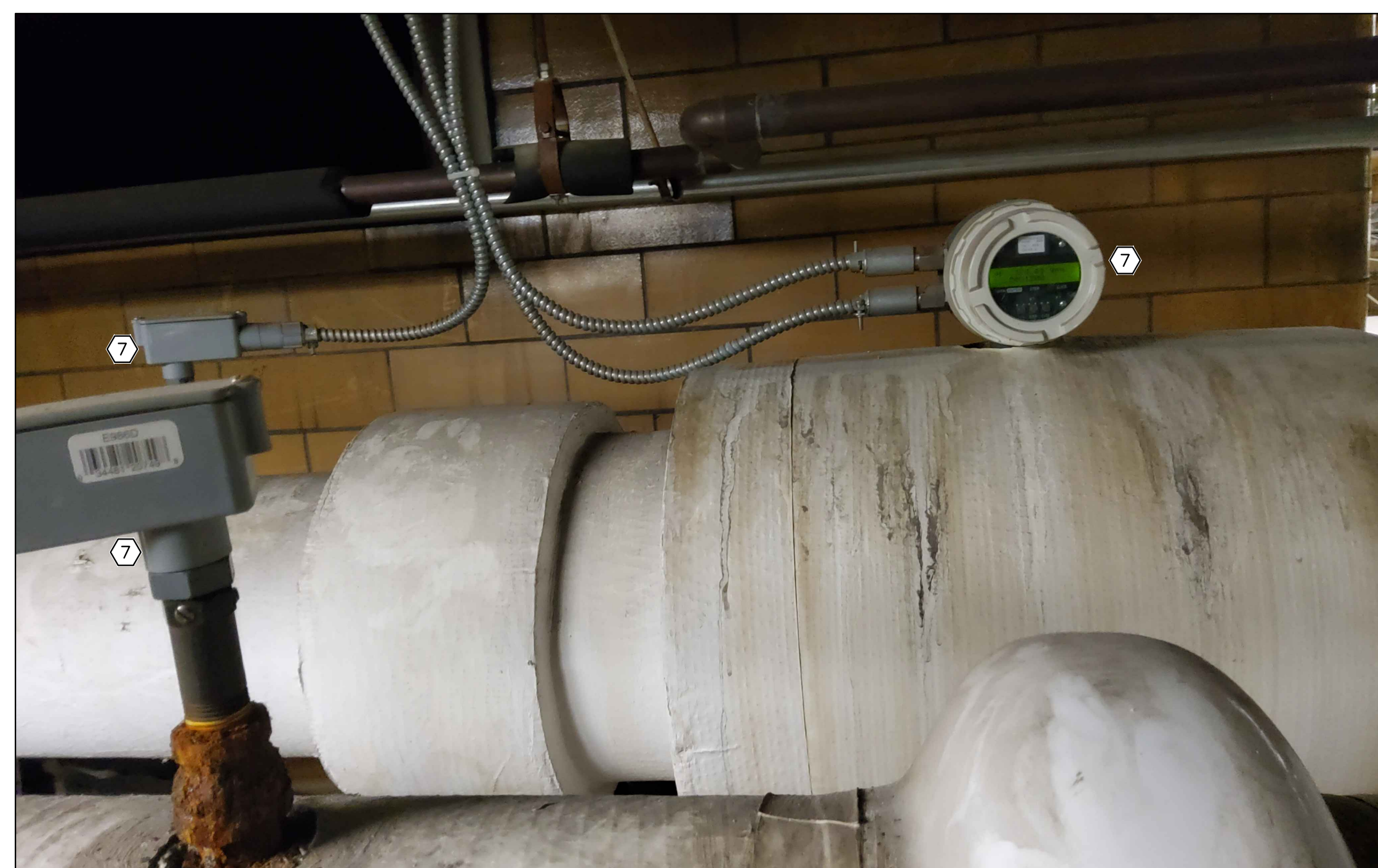
8 PHOTO: CHILLED WATER METER AND TEMP SENSORS TO BE DEMOLISHED M-5 Scale: NONE
