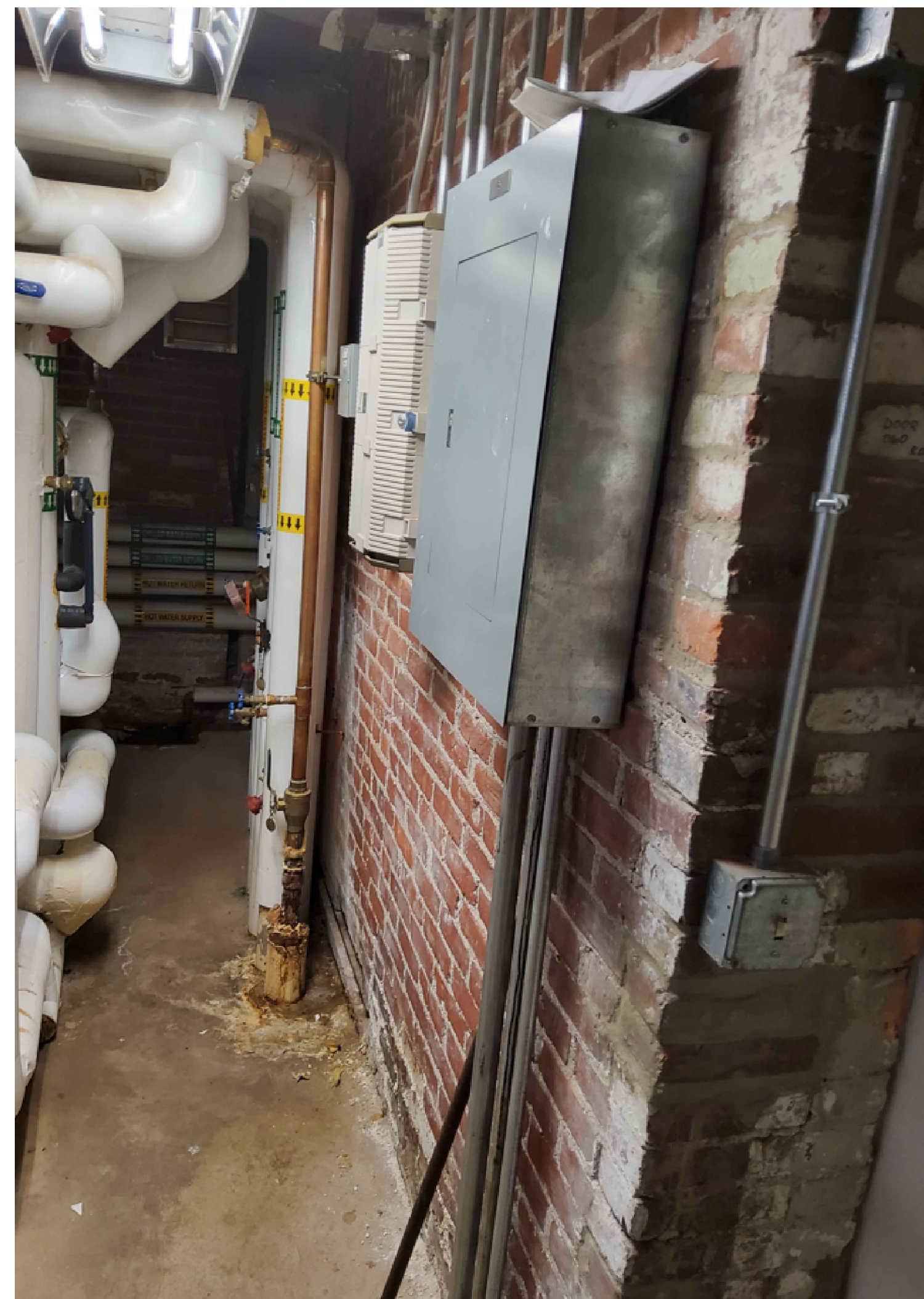
4 M-12 PHOTO: EXISTING JCI PANEL IN WATER SERVICE ROOM Scale: NONE PROVIDE NEW CONTROL PANEL ADJACENT TO EXISTING
