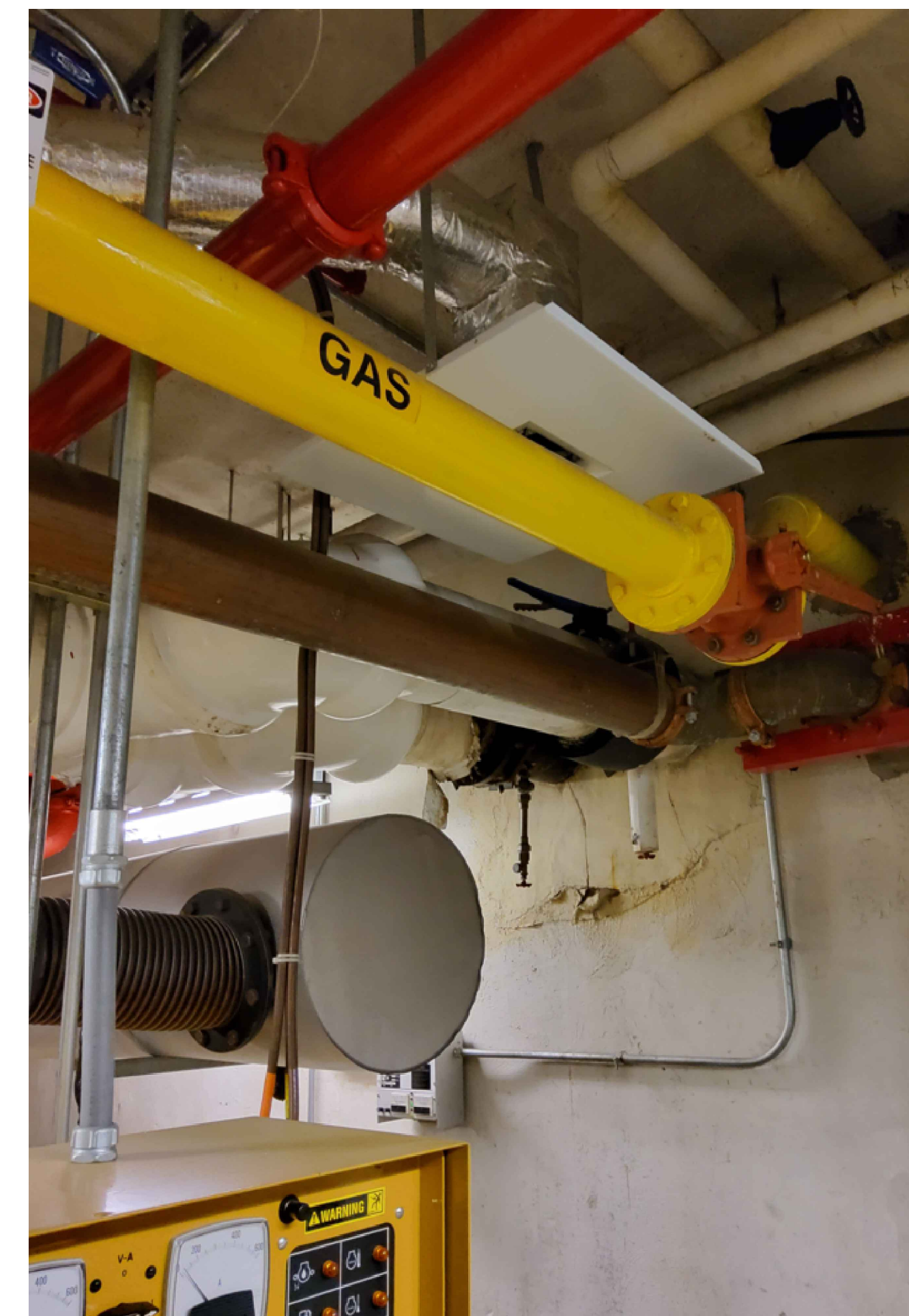
5 PHOTO: GAS SERVICE ENTRANCE Scale: NONE LOCATION OF METER
