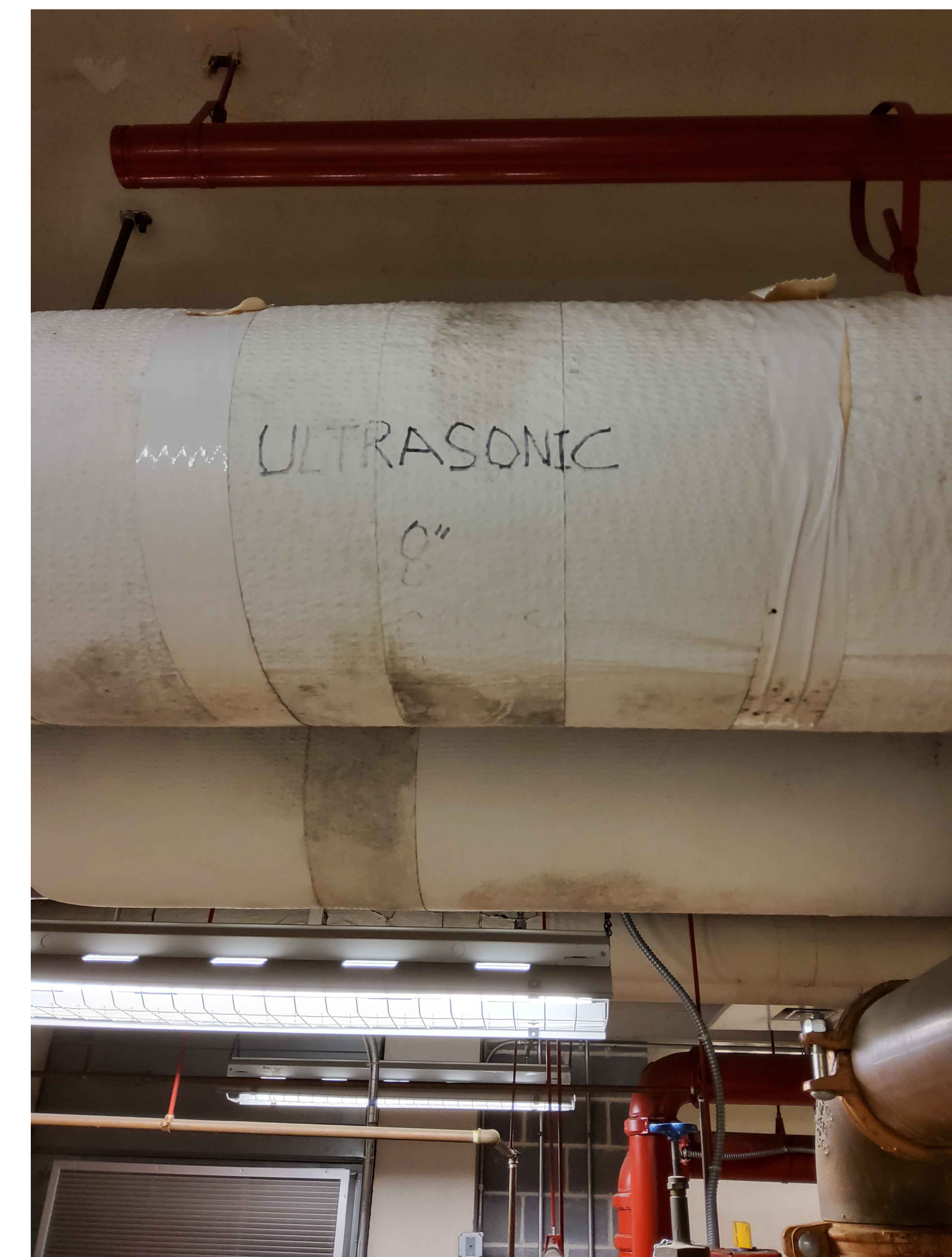
7 PHOTO: CHILLED WATER PIPING Scale: NONE
