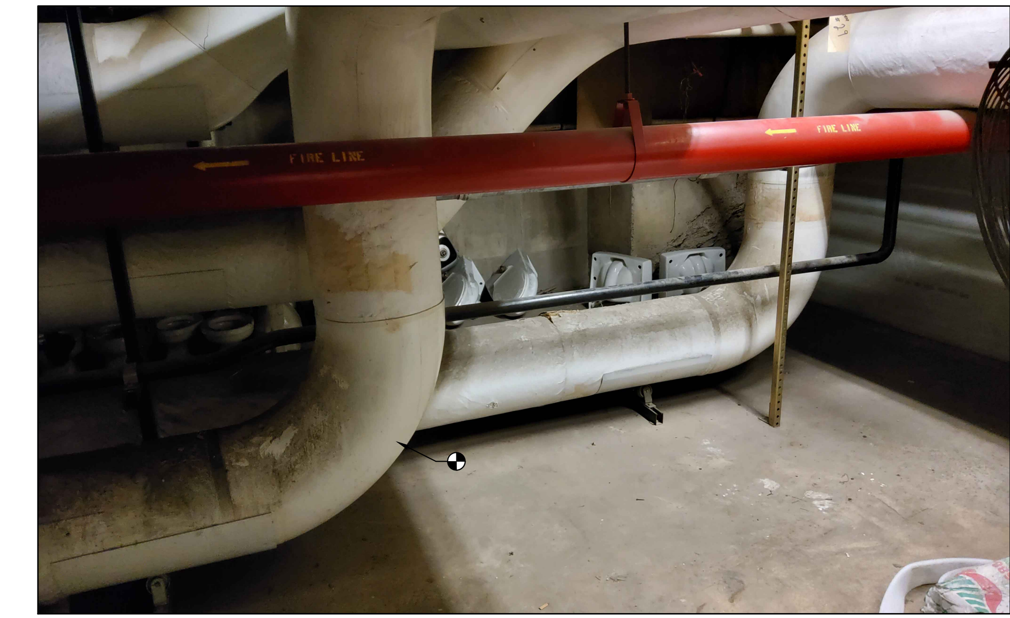
7 M-9A EAST (CENTRAL CHWS) Scale: NO SCALE SERVES EAST AND MAIN CAPITOL
