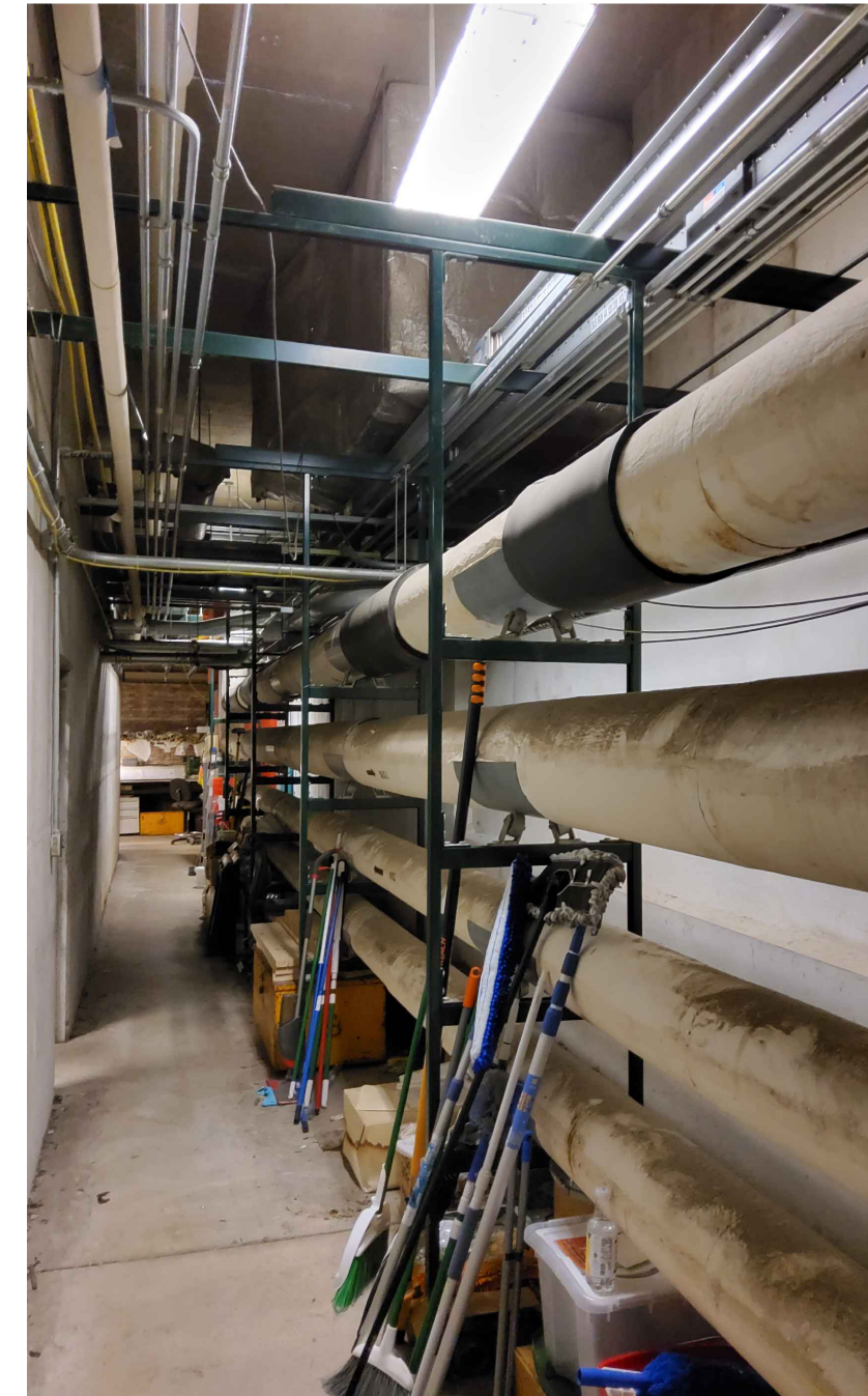
3 PHOTO: CHWS METER LOCATION M-10 Scale: NONE NORTH SIDE OF BUILDING
