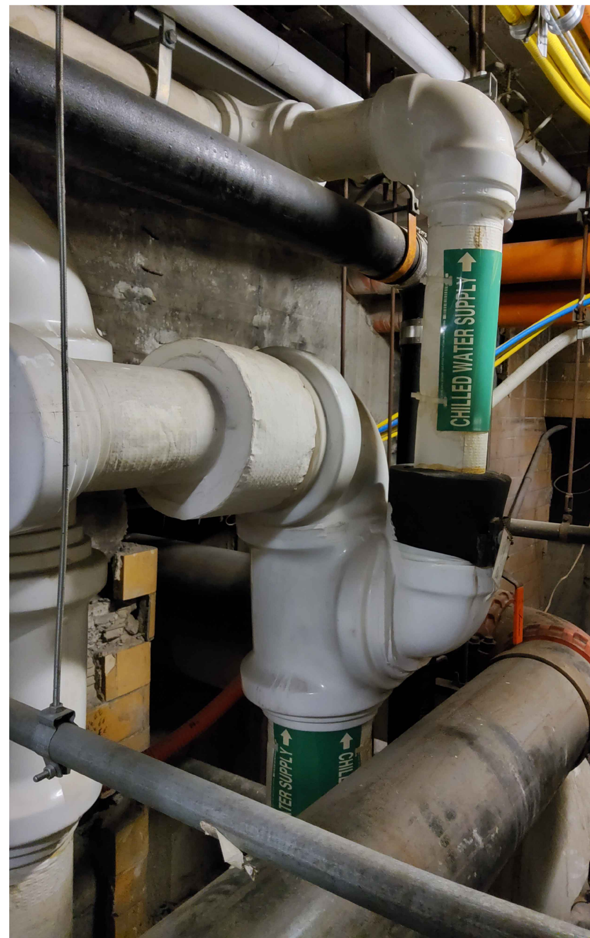
4 PHOTO: LOCATION OF NEW CHWS METER M-8A NOT TO SCALE SENATE NOB-CHWS-M02
