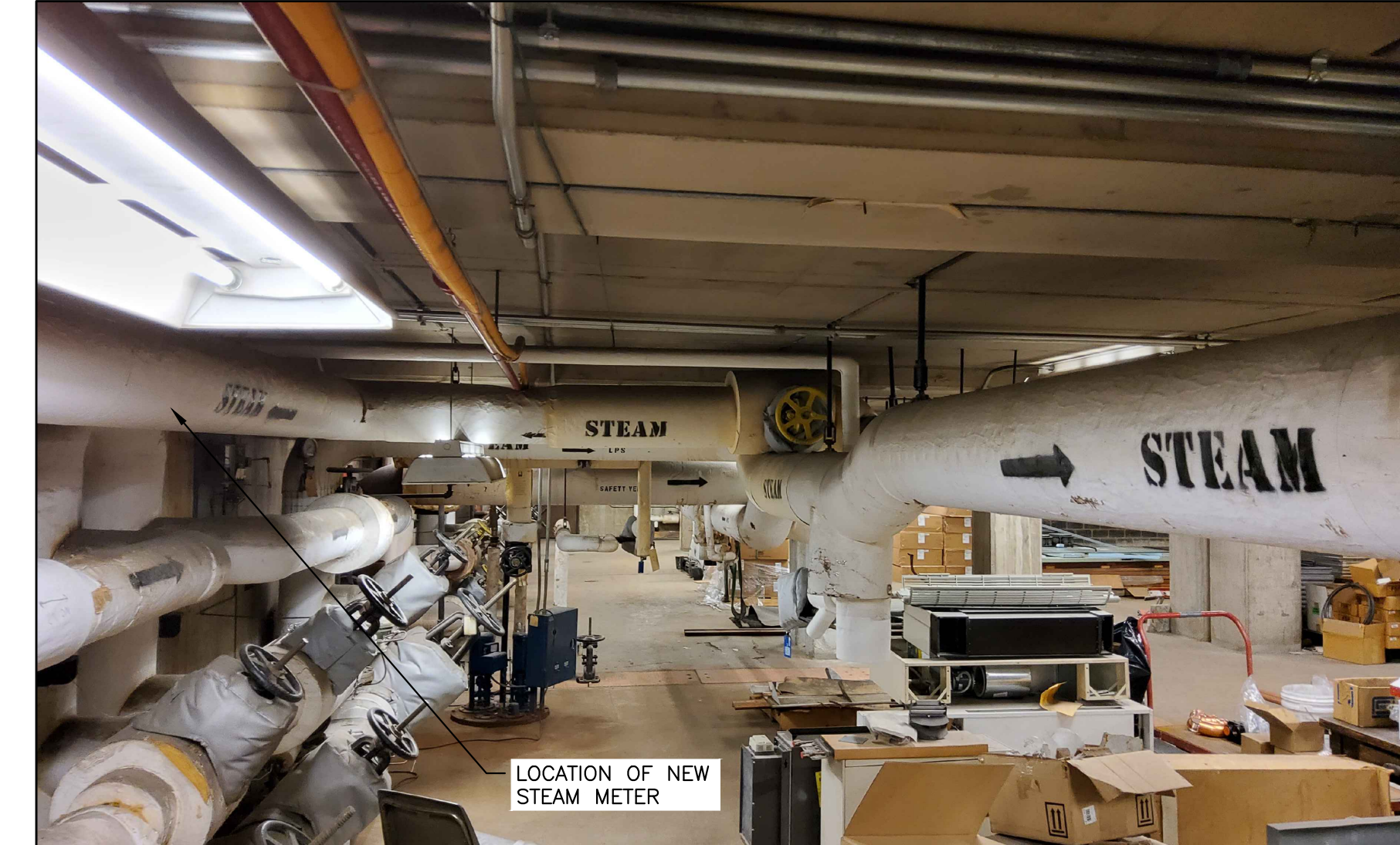
5 PHOTO NORTH STEAM M-9B Scale: NONE SERVES EAST BLDG NORTH
