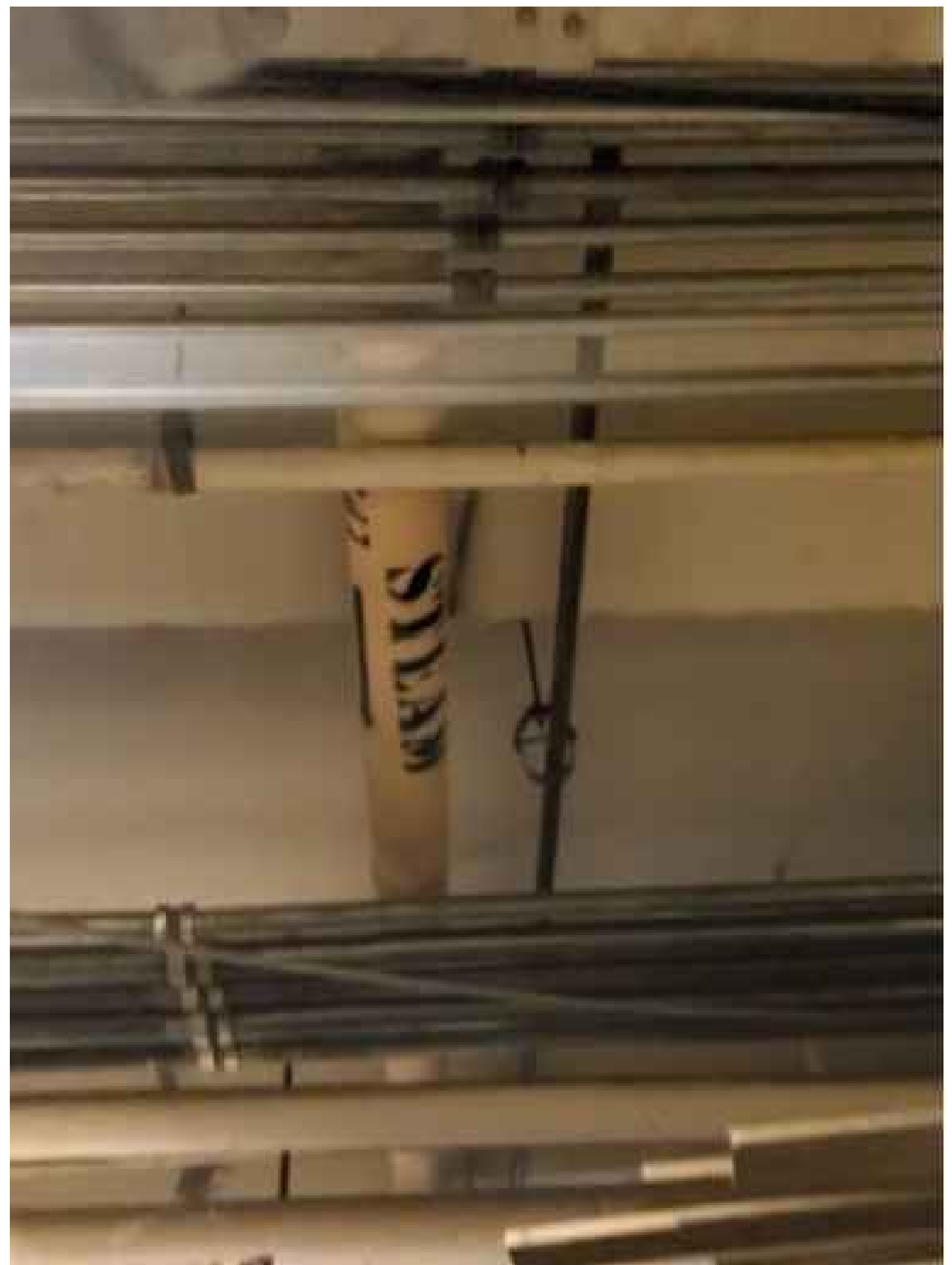
5 PHOTO: LOCATION OF NEW STEAM METER M-8A NOT TO SCALE NOB-STM-M02 FOR DOMESTIC HOT WATER
