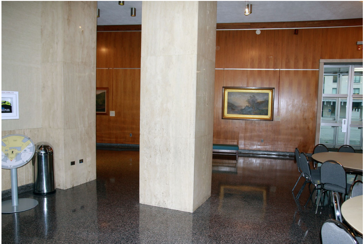
Photograph 3 Northeast corner of Memorial Hall 114 showing examples of terrazzo floors and travertine outside corners to be protected.
