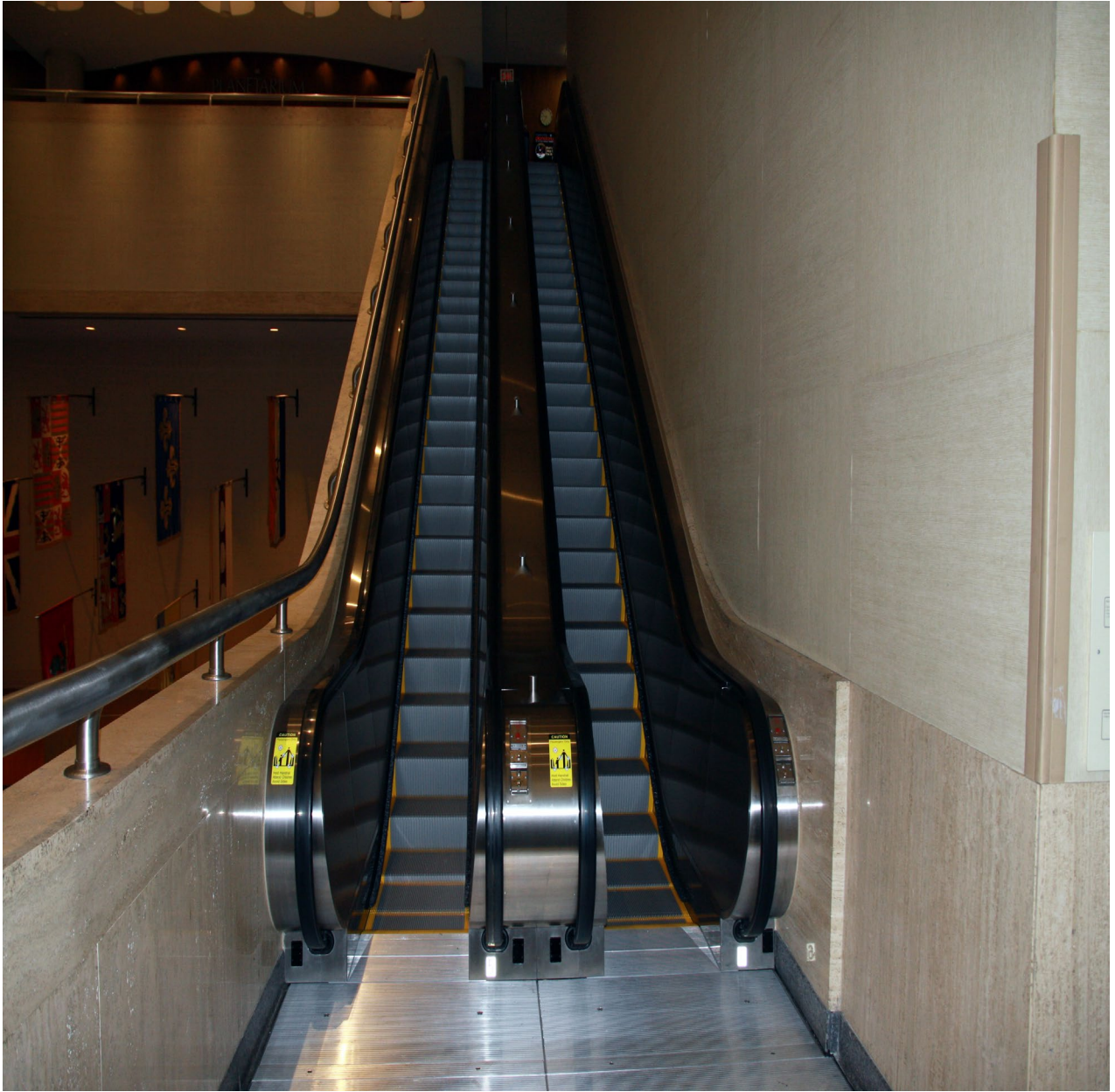
Photograph 4 Escalators 3 and 4, as well as the other four escalators, have been recently modernized. The escalators shall not be used by construction personnel.
