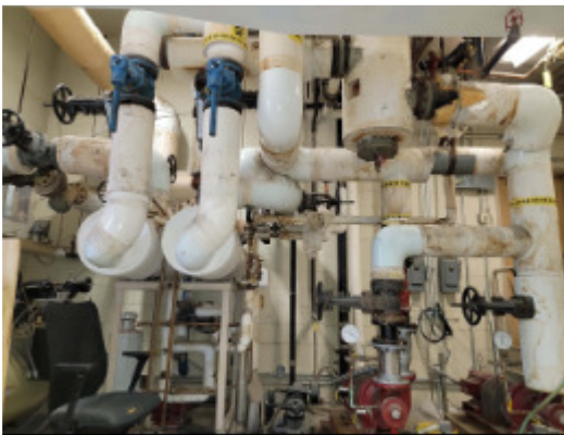
Mechanical Room 171 Overview
