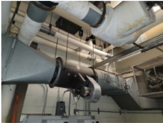
Mechanical Room 171 Overview
