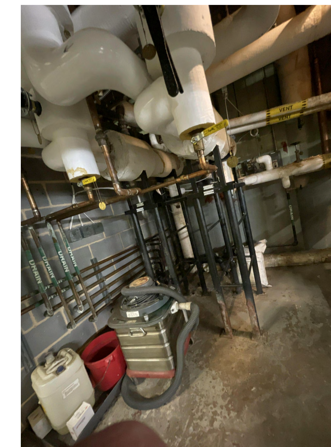
1 MECHANICAL ROOM BB12 - EXISTING HPS ZONE VALVES NTS
