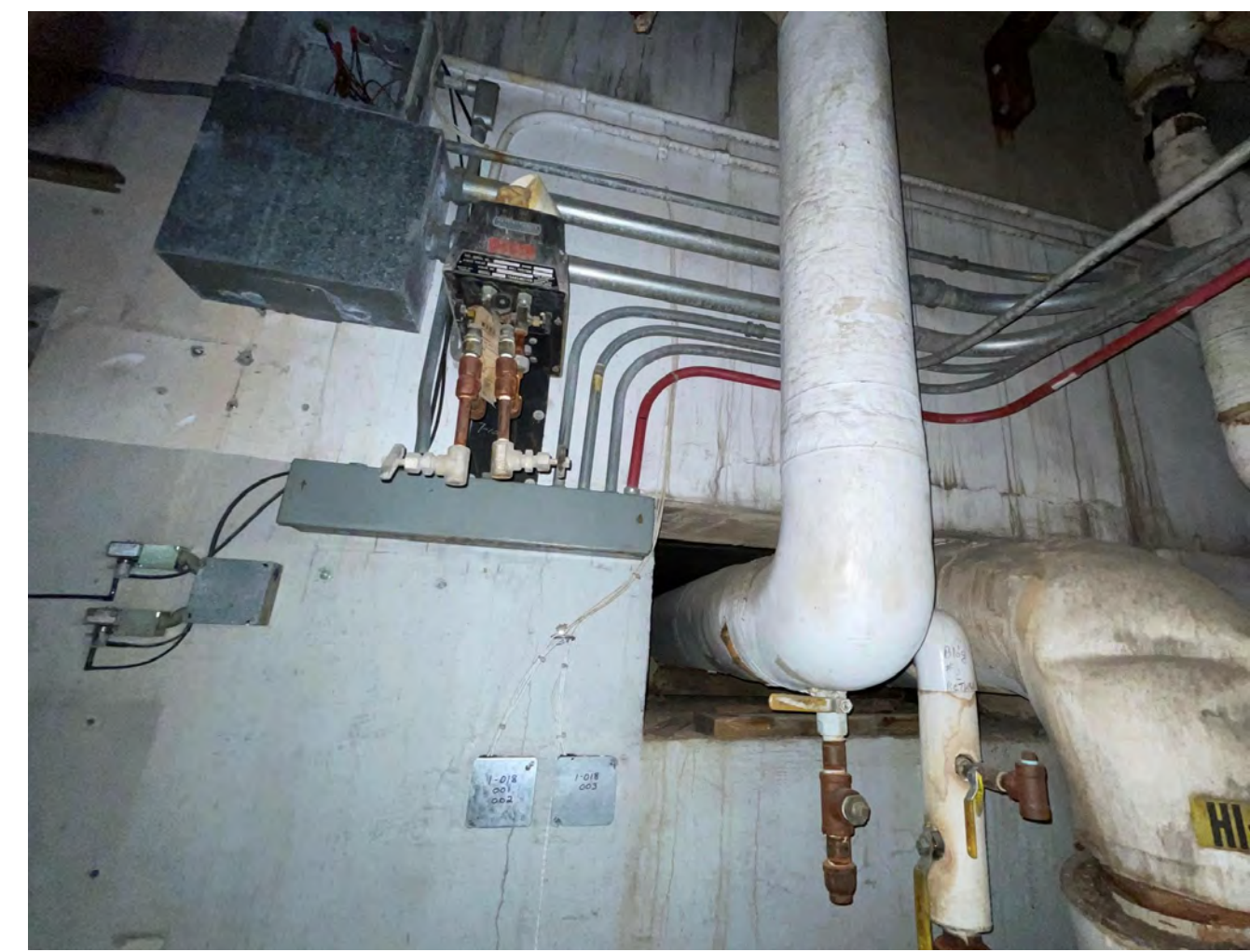
8 MECHANICAL ROOM BA10 - EXISTING PNEUMATIC CONTROLS EXAMPLE NTS
